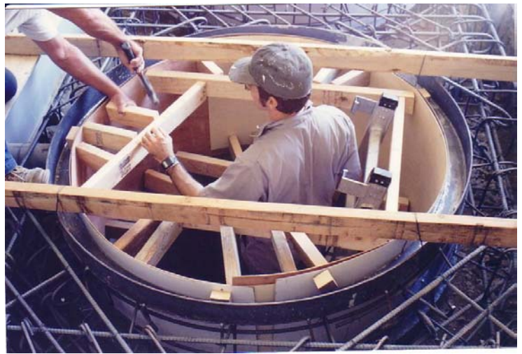
The safest place for cryostats may be underground. Underground vaults from reinforced concrete provide protection against many hazards.
